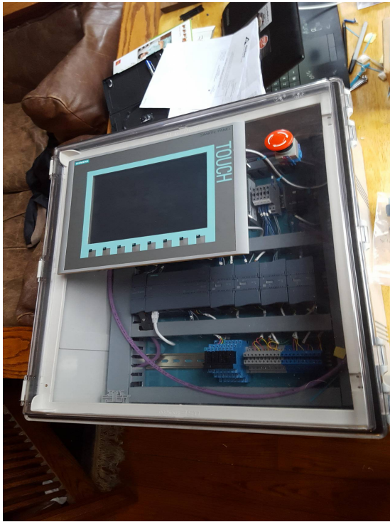
Figure 15. S7-1215 mounted with see through for I/O status. IP63
